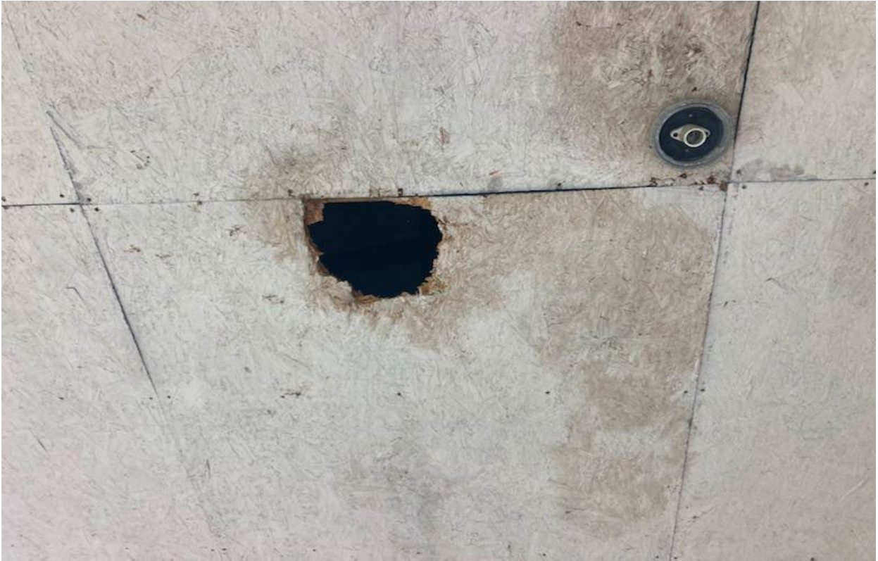
Holes in the ceiling of the pavilion at Robvanary Park.
